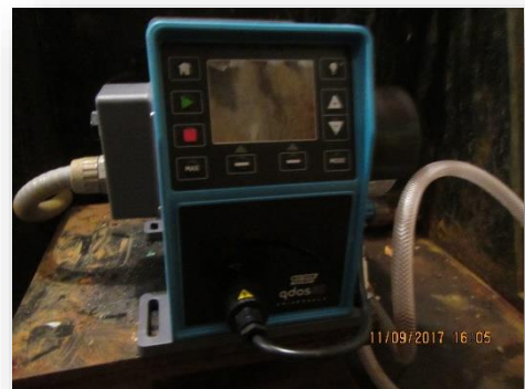
FIGURE 7 NEW FERRIC CHLORIDE PUMP
